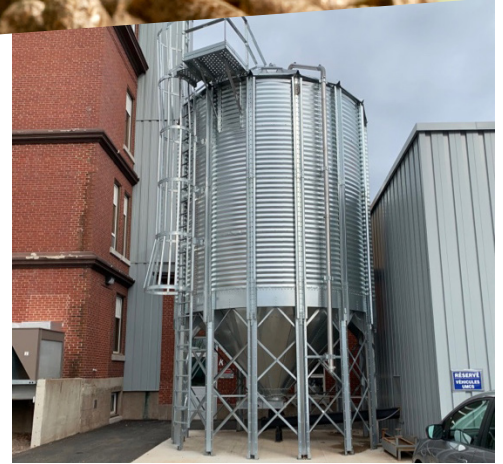
The farm-style silo holds approximately 30 tonnes of pellets and is refilled every 20 days in the height of winter.
