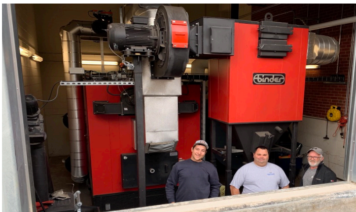
Serge Mallet, responsible for mechanical/electrical systems and buildings maintenance at the CCNB-UDM Shippagan Campus seen here with colleagues Sebastien Chiasson (left) HVC Mechanical and janitor Maurice Gagnon (right).
